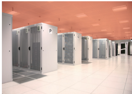
Ceiling protection at Data center
