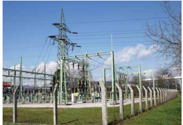
Perimeter protection X Laser scan / Outdoor PIR detectors
